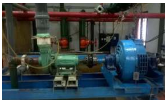
Photo No. 01: Pumps used as Turbines in test rig.
